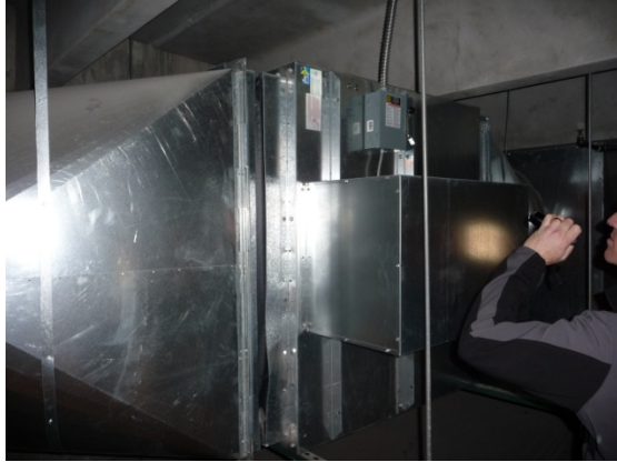
Fig. 3: Garage large exhaust fan
