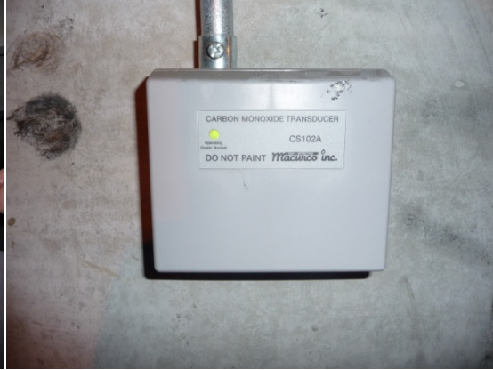
Fig. 4: Garage CO wall sensor
